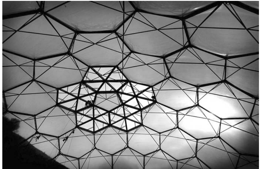
A biome nearing completion as the last of the foils are put into place. The biomes were constructed around the biggest free-standing scaffold structures ever built.
