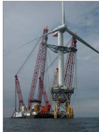
Courtesy - Talsman / Scaldis REpower 5MW turbine being installed on Beatrice Project in 44m of water on a jacket structure. Rotor - 126m diameter Tower, nacelle and rotor installed in one lift as pre-assembled unit
